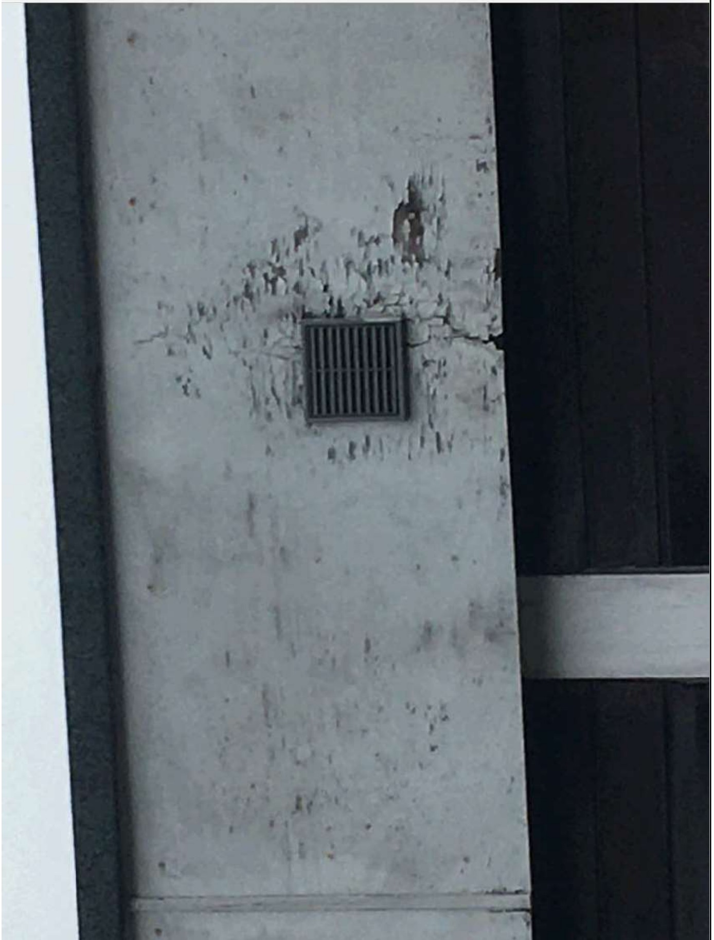
Image shows cracks to the building and its general condition
